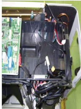
Replace New PCB
